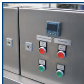
Process water temperature control via individual controller
